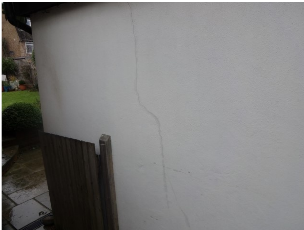
Cracked render to left hand side of kitchen
