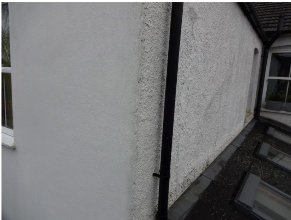
Cracked render to bedroom 412DUPLICATE Name - Change position
