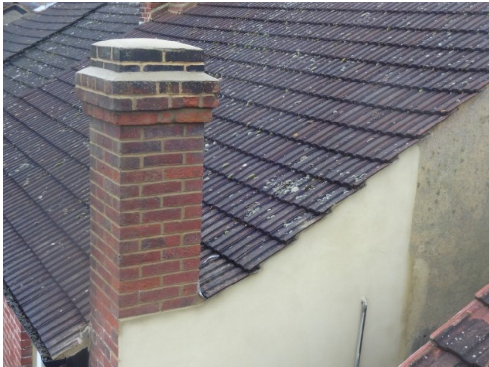
Front bedroom chimney capped stack Change position
