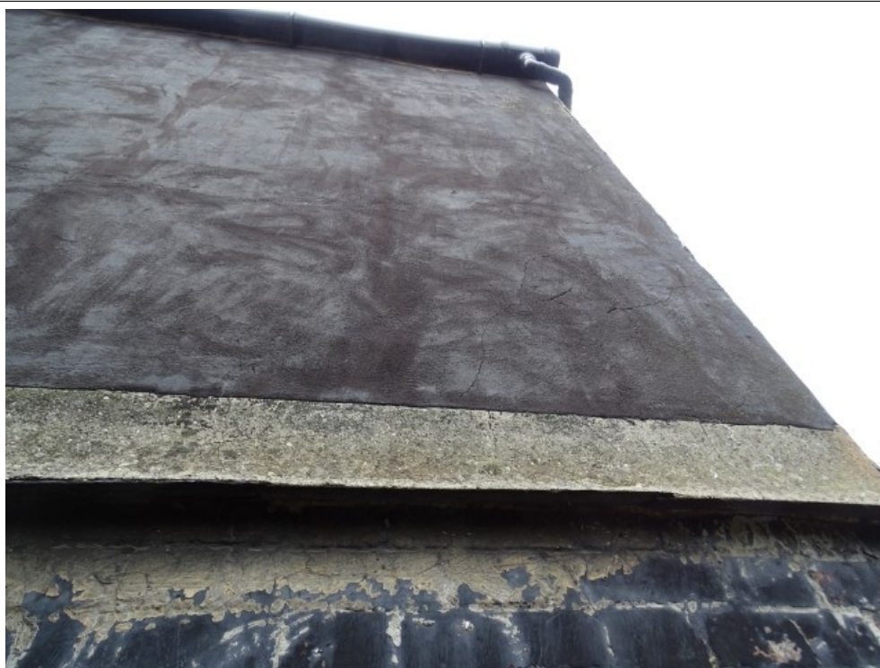
First floor rear gable wall cracks in render
