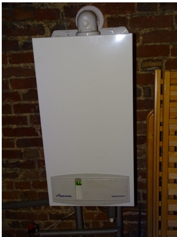
Gas boiler in loft
