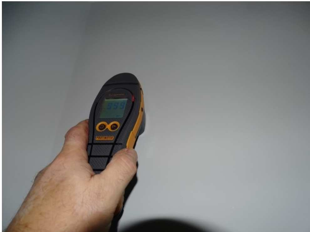
Dampness to front small bedroom to side of chimney
