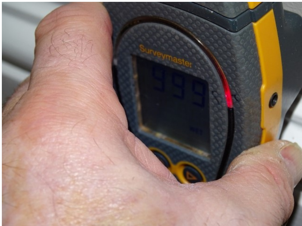
Dampness to front wall of sitting room
