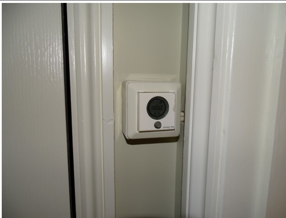
Room stat to underfloor electric heating
