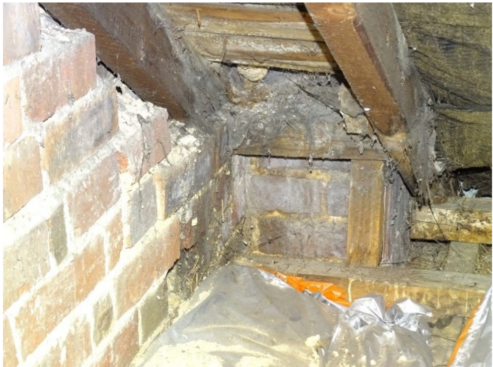
Chimney stack from small front bedroom showing dropped sarking felt
