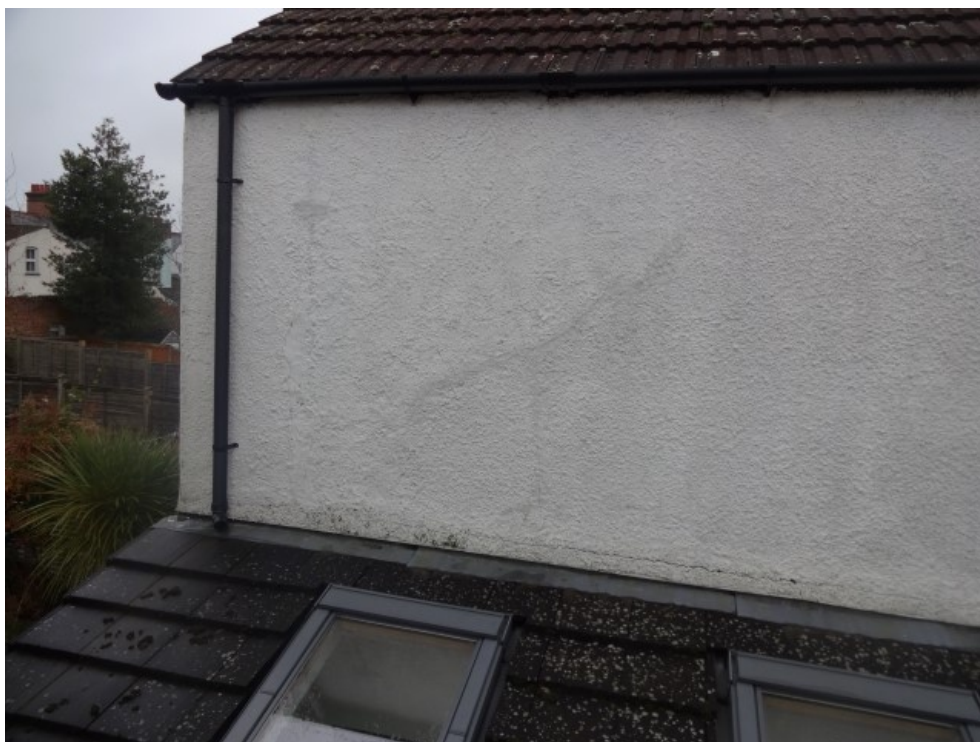
Cracked render to bedroom 4
