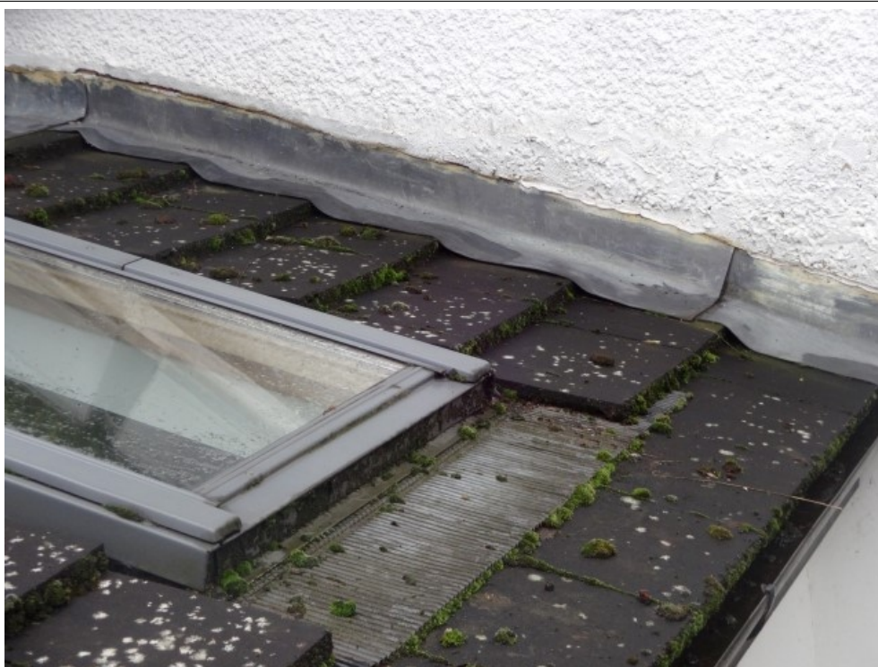
Render cracking above lead flashing onto roof of dining area
