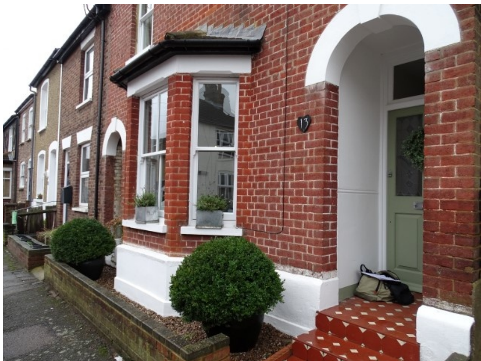
Front wall to right hand side of bay window wet
